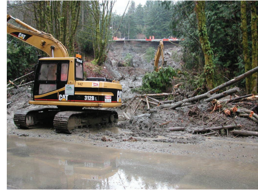
Landslide on U.S. 101 northwest of Olympia. Photo by Karl Wegmann (DNR)
