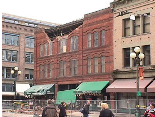
URM brick wall failure at historic Cadillac Hotel, Seattle. Photo by A. Sanli and M. Celebi (USGS), S. Akkar (METU)
