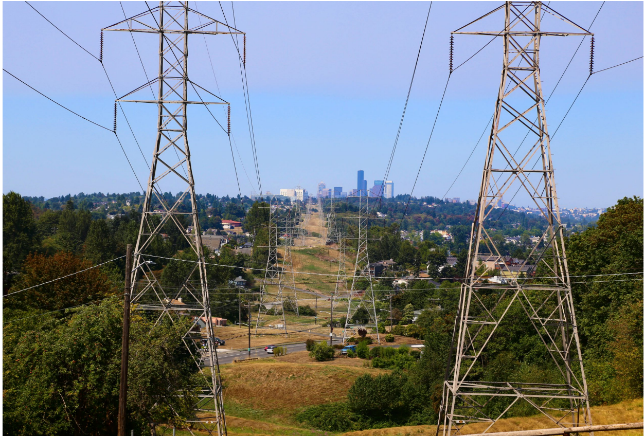
Seattle City Light transmission lines overlooking downtown Seattle.
