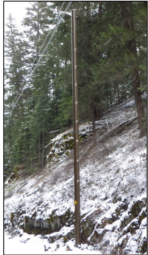
Figure 28: Distribution Fiberglass Poles
