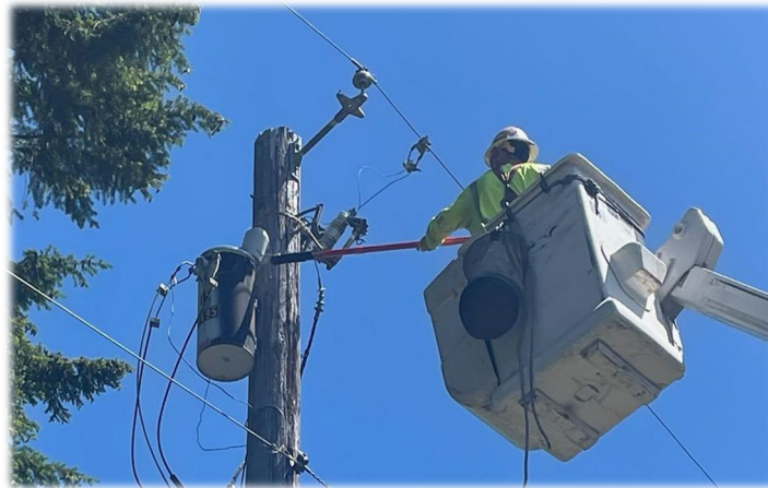
Figure 1 - Overhead Transformer Installation
