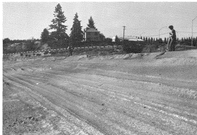
Figure 27.—Yakima's Chesterly Park ash landfill. Five-acre site containing 90,000 cubic yards of ash.
