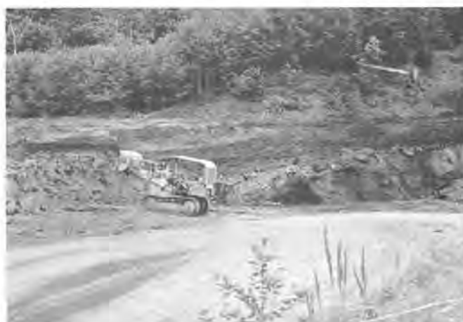
FIGURE 34.— Stripping overburden off the clay seam at the Harris deposit, in King County, Washington. Front-end loader is on minable clay.
