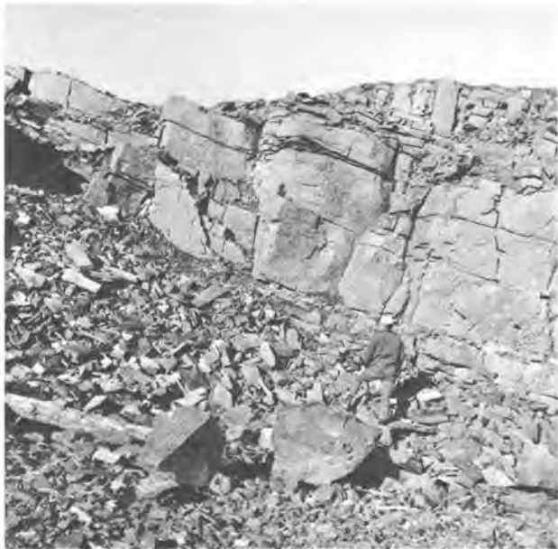
FIGURE 70.— Jointing in basalt of the Fall City stone quarry, in King County, Washington.
