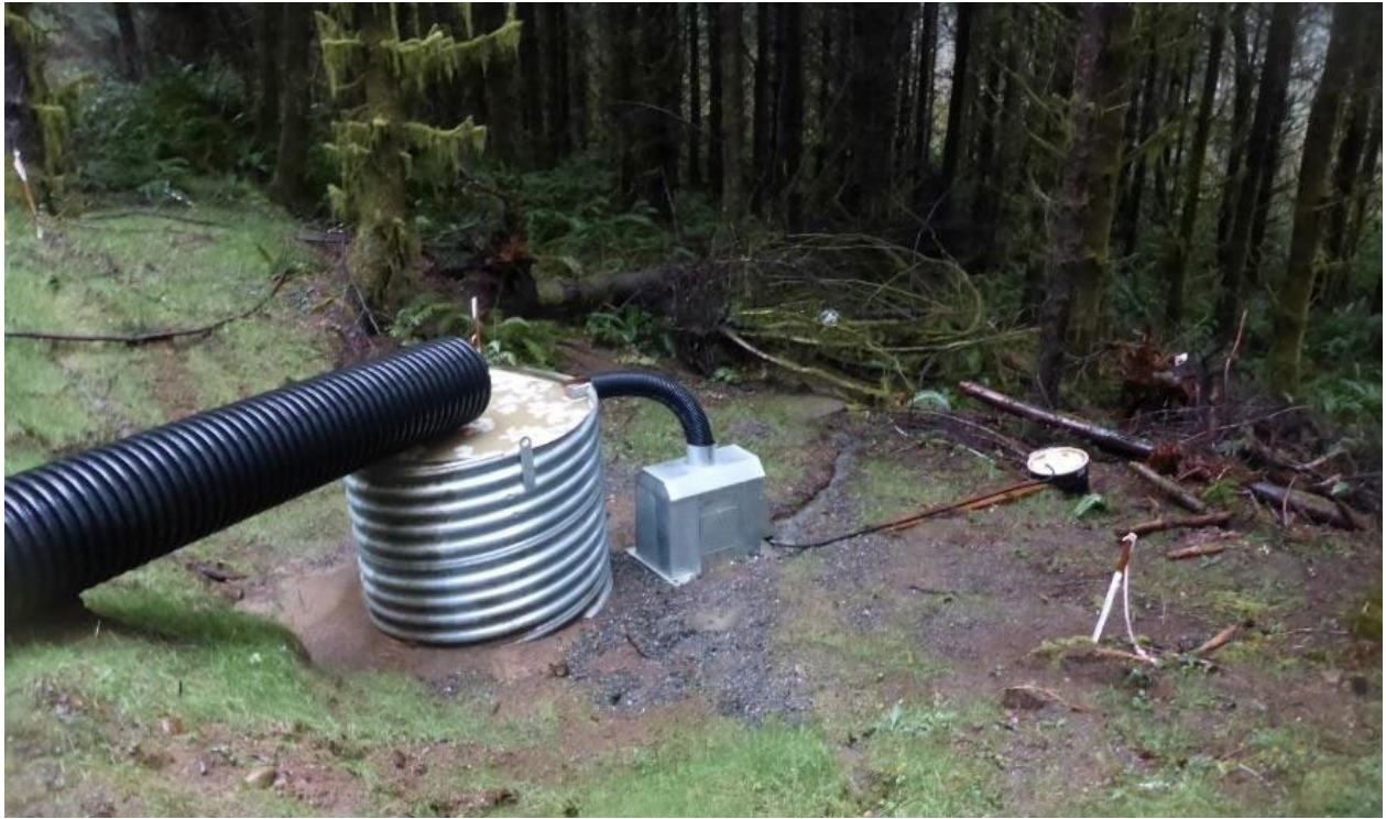
Figure 2: Field data collection setup. The upper figure shows the road surface routing water to the ditch and the collection trough. Water and sediment then are routed through a culvert pipe to the sediment tub. The lower figure shows the platform with the sediment tub collecting road sediment, the tipping bucket measuring discharge and the suspended sediment tank(SST) sampling the fine sediment that is not settled in the tub.
