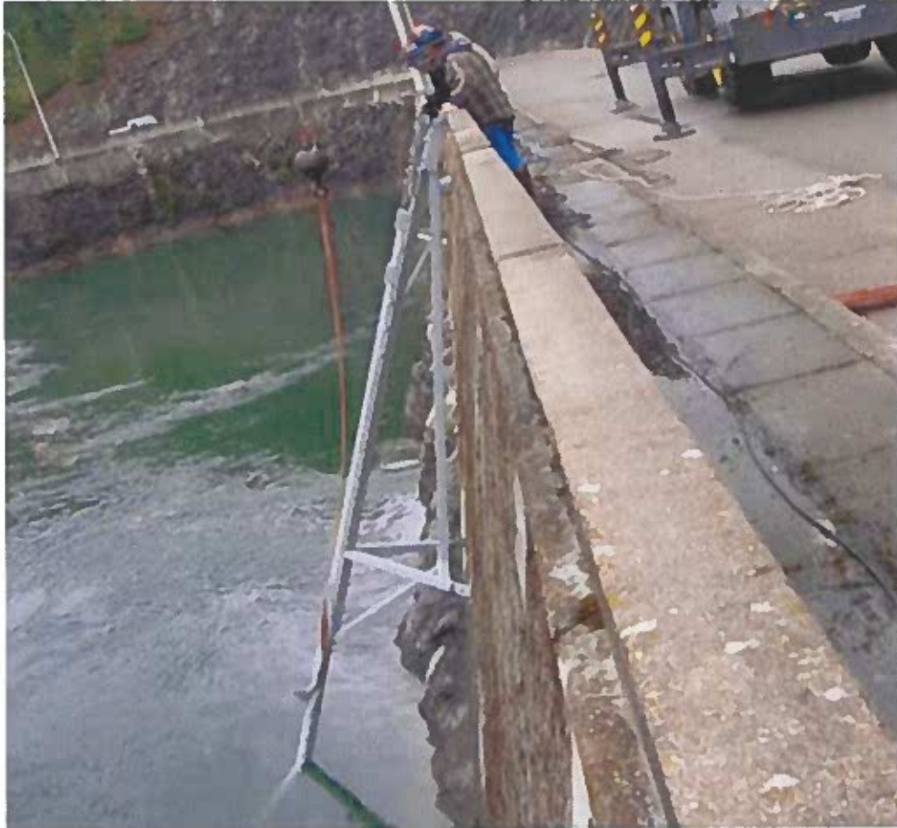
Figure 5. Intake Forebay #7 hydrophone mount deployed for the Boundary Project telemetry project.
