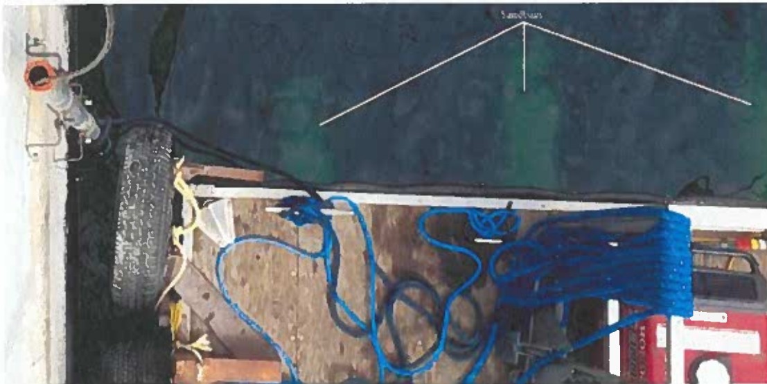
Figure 7. Overhead view of the above water section of the Spillway West #5 hydrophone cable conduit attached to the parapet wall upstream of Spill Gate 1.
