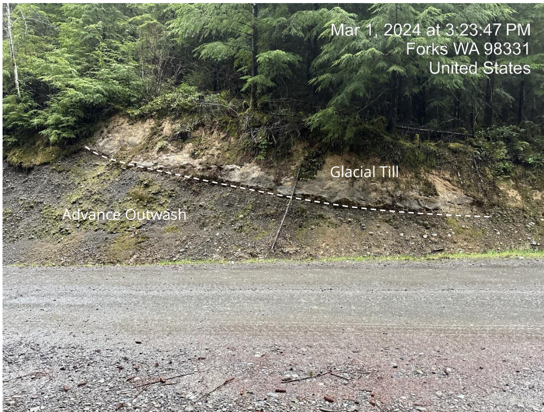
Image 10. Roadcut showing backrotated contact in the head of the landslide
