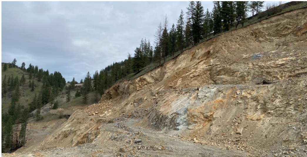
VIEW LOOKING NORTH AT THE TOPPLED ROCK DEBRIS AND OVERSTEEPENED WALL AT CUT 2. THE DETACHED BEDROCK ALONG BEDDING LEFT A PROMINENT PLANAR SURFACE. START OF CUT 3 VISIBLE AT RIGHT.
