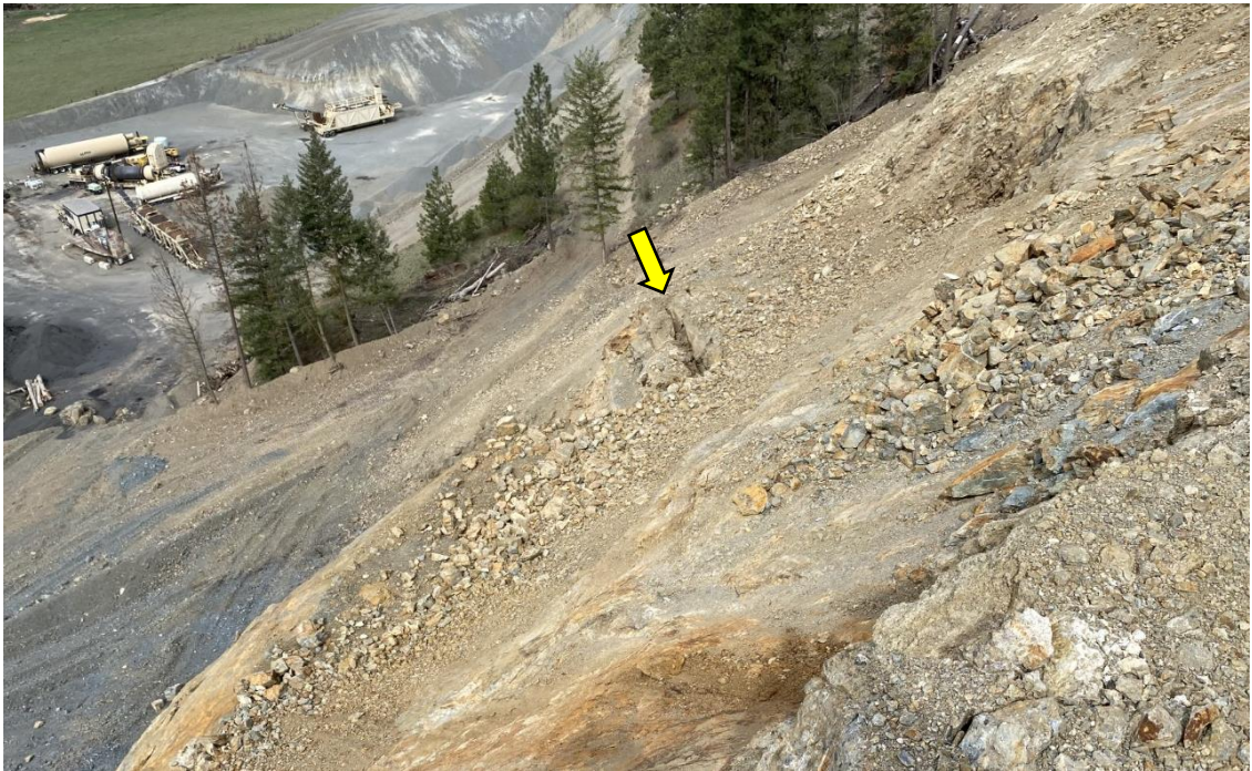
BEDROCK CRACK (YELLOW ARROW) OBSERVED IN THE MIDDLE OF THE HIGHWALL IN CUT 1. THIS CORRESPONDS TO THE CRACK MAPPED FURTHEST NORTH ON FIGURES 2 AND 3. VIEW IS TO THE NORTHWEST.
