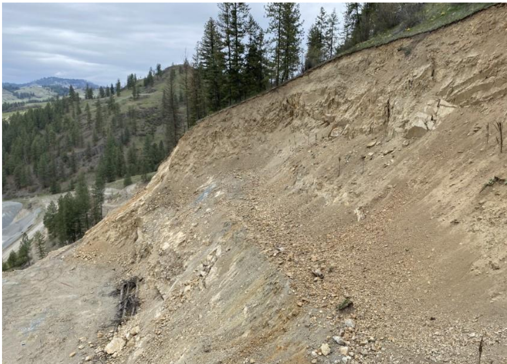
VIEW NORTHWEST OF THE HIGHWALL AT CUT 3. THE HIGHWALL GRADIENT IS LESS STEEP THAN THE OTHER TWO CUTS – THOUGH STILL STEEPER THAN 2H:1V – AND APPEARS TO INCLUDE AT LEAST TWO RELICT BENCHES.
