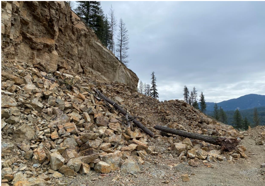
OVERSTEEPENED WALL AND ACCUMULATED ROCK DEBRIS ON THE BENCH AT CUT 2. VIEW IS TO THE SOUTH.
