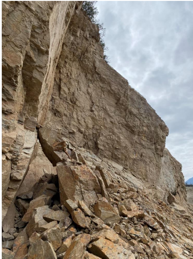
OVERSTEEPENED WALL AT CUT 2. NOTE THE FLAT, TABULAR PARTINGS IN THE BEDROCK FROM HIGH-ANGLE ROCK JOINTS. VIEW IS TO THE SOUTHEAST.
