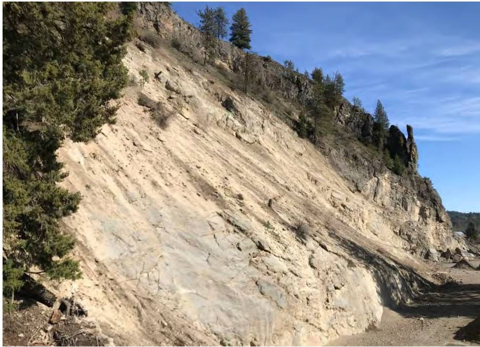
VIEW PARALLEL TO THE MINED EXCAVATION, INCLUDING THE TALUS SLOPE UNDERLAIN BY A BEDROCK CUT IN THE FOREGROUND, AND THE BEDROCK EXCAVATION WITH ROCKFALL IN THE BACKGROUND. PHOTOGRAPH TAKEN FACING SOUTH/SOUTHEAST. NOTE THE NATURAL OUTCROP ABOVE BOTH SLOPES ORIENTED PARALLEL TO THE BEDDING EXPOSED IN THE BEDROCK EXCAVATION. ROCK PINNACLE ALSO VISIBLE AT THE RIGHT END OF THE NATURAL OUTCROP.
