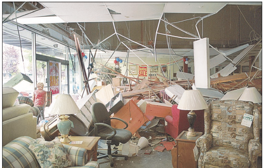
Figure 2. Merchandise inside Moore's Furniture in Aberdeen, Wash., lies smashed after a 5.9 magnitude earthquake struck the area July 2, 1999. Extensive damage to the Moore's building was caused by an exterior wall that collapsed inward, crashing through the ceiling of the furniture store. Photo and caption courtesy of Kevin Hong, The Daily World, Aberdeen, Wash.
