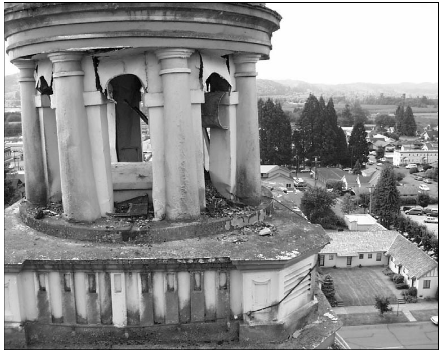
Figure 1. Cupola of the Grays Harbor County Courthouse in Montesano, Wash. This historic building suffered several million dollars' worth of damage during the July 2 earthquake whose epicenter was about 1 mile away. Photo and caption courtesy of Grays Harbor County.
