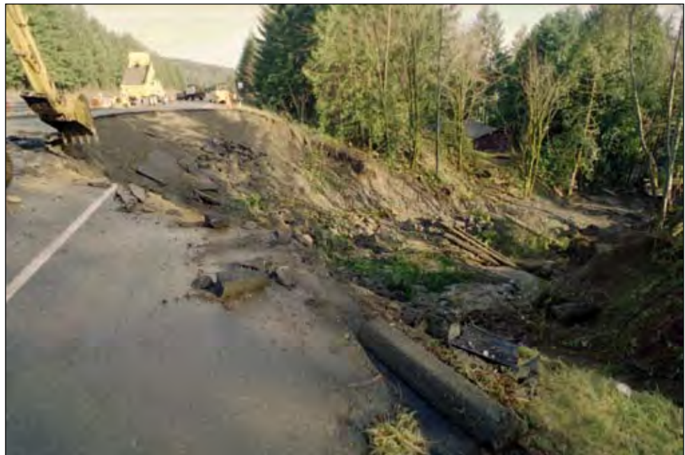
Liquefaction, lateral spreading, and landslides damaged many roads throughout the area. Photo: William S. Lingley, DGER
