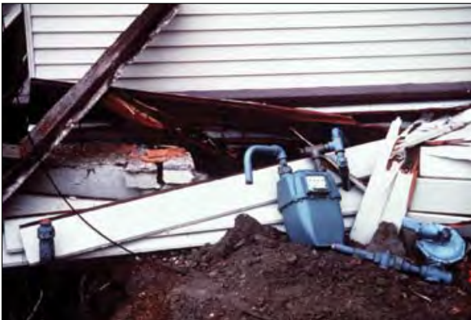
This house shifted off its foundation, breaking the utility lines and leaving it uninhabitable. Newer building codes require a house being tied to the foundation, but homeowners may need to retrofit older homes. Photo: USGS
