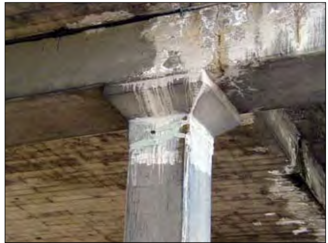
The South Park Bridge in Seattle suffered extensive damage. Above is one of 22 columns that cracked in the earthquake. Epoxy was injected to shore up the structure. Crews worked round the clock to repair this and other structures throughout the area. Photo: King County
