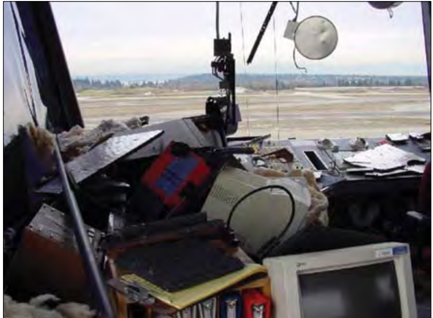
The tower at Sea-Tac sustained both structural and nonstructural damage. Even so, the airport was able to reopen after a few hours. Photo: Washington State Department of Transportation
