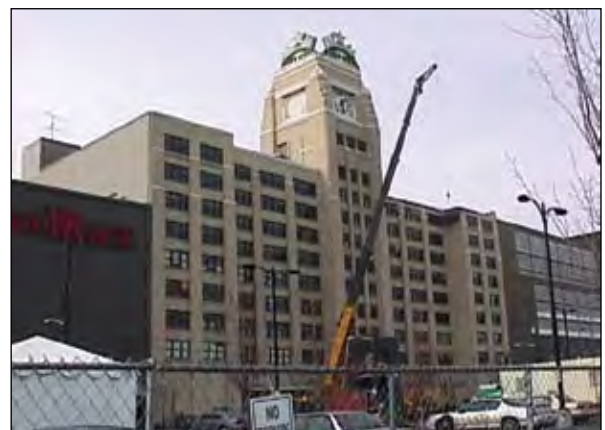
Earthquake retrofits and other preparations paid off at the SODO Center for Starbucks. They were able to sustain the interruption due to the earthquake. Photo: A. Sanli and M. Celebi, USGS; and S. Akkar, METU, Turkey
