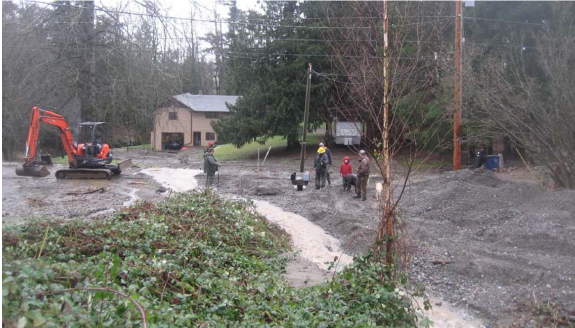
Figure 9 View of area along Goodwin Road in front of 6488 and 6500. Stream is essentially flowing in same location as prior to debris flood event. However, stream is now several feet above original channel. Residence at 6489 Goodwin Road in background. Debris flowed over surface in front of house and into an area to the right. View looking westerly. Photograph taken 1/8/09. (Photo by D. Hooks)
