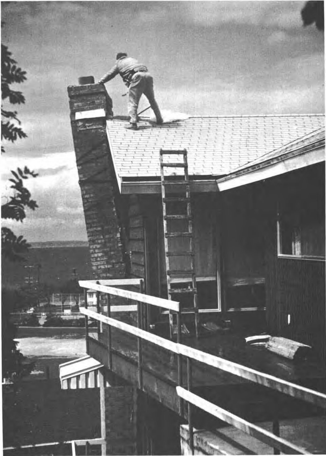
Figure 20.—Chimney damage in West Seattle. (Photo by Karl V. Steinbrugge.)
