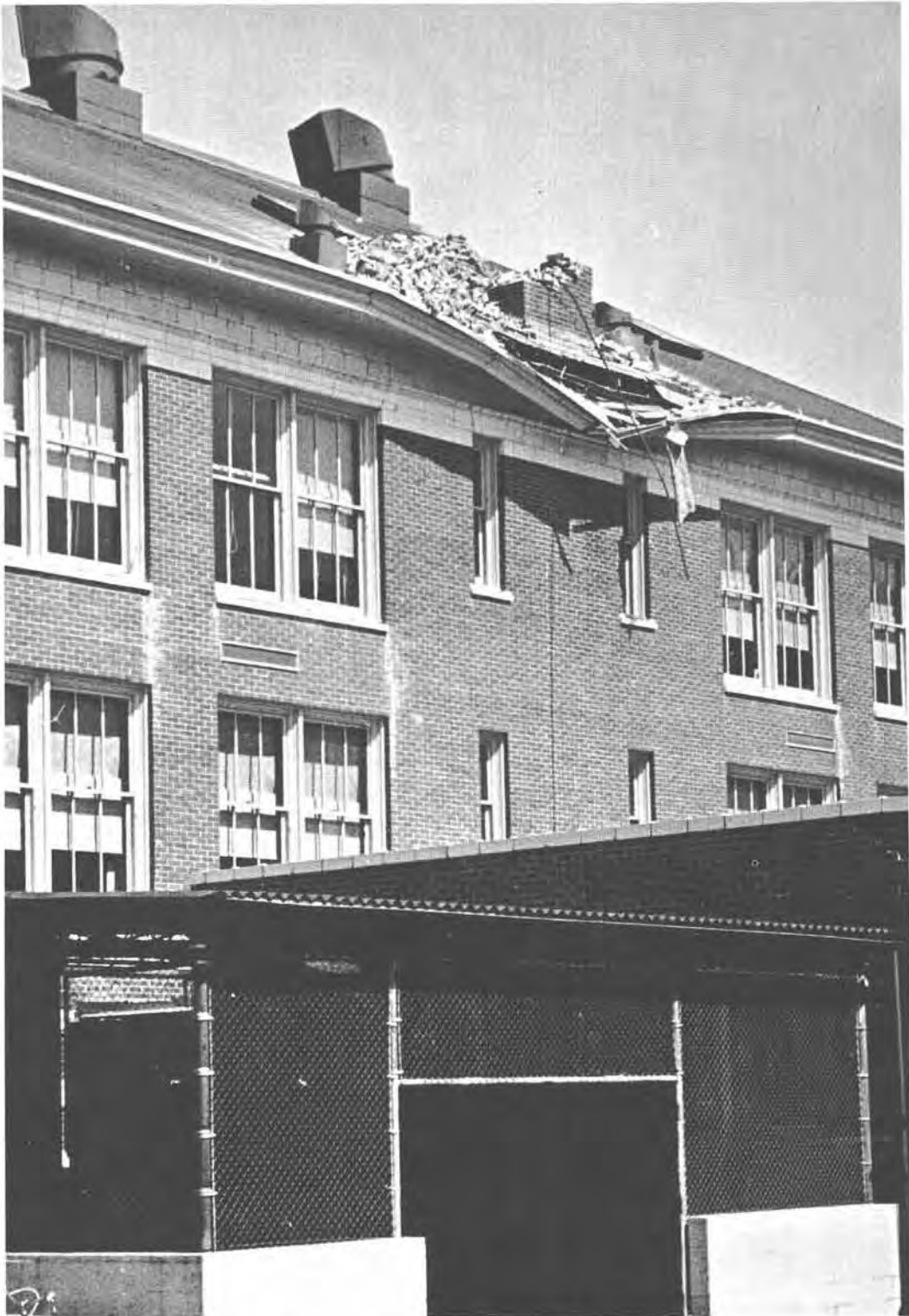
Figure 18.—The 60-foot brick chimney at the Alki Elementary School in Seattle collapsed on the one-story boiler room, severely damaging it. (Photo by Cory Tolman, Seattle Post-Intelligencer.)
