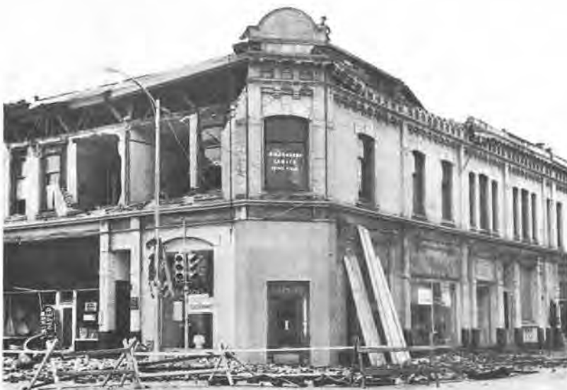
TOP—Poorly anchored brick veneer was knocked off Seattle structure. The obvious lesson here is that building facings must be designed to resist a reasonable amount of horizontal force.
