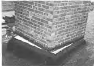
MANY UNREINFORCED masonry chimneys were fractured and rotated far more than this one, which gave way at the flashing point above the roof. A competent designer could have avoided this weakness.
