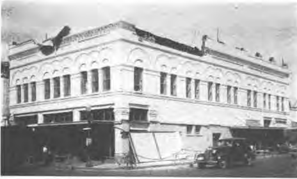
FIG. 9—Olympia. Parapet wall was knocked off and carried a canopy to the sidewalk with it.
