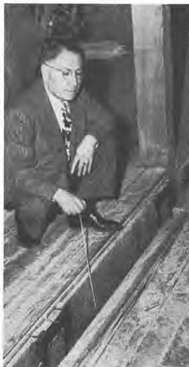
WATERFRONT STRUCTURES supported on piles driven into fill material shows a differential settlement of 8 in. on the fill side.
