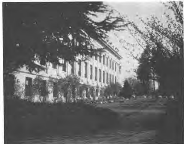
FIG. 13—State Insurance Building, Olympia. Heavy stone ornamental parapet was thrown off for the entire length of the building.
