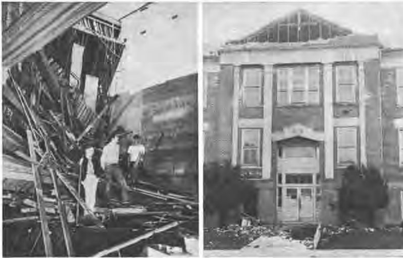
LEFT—Unanchored roof and ceiling beams over the stage of Puyallup high school auditorium slid off supporting masonry walls and crashed to floor, causing $100,000 damage.
