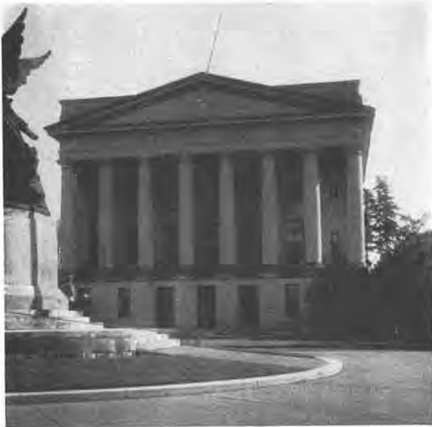
FIG. 12—State Insurance Building, Olympia. Stone cornice at upper righthand corner was shoved out and ready to collapse.
