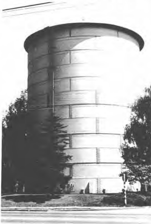
Figure 27.—Woodland Park Standpipe, Seattle. Typical damage to anchor bolts may be seen in next figure. (Photo by Washington Surveying and Rating Bureau.)
