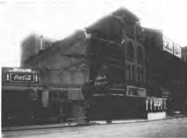
FIG. 1—Parapet wall of the second story wall fell due to lack of anchorage and inferior masonry.
