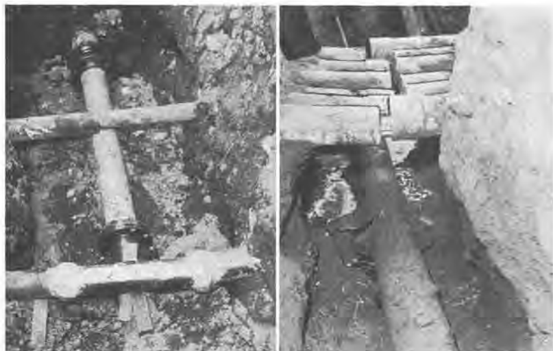
LEFT—Water and sewer lines fractured with pollution inevitable unless break is uncovered. RIGHT—Movement in soft ground pulled open these conduits in spite of locknuts.
