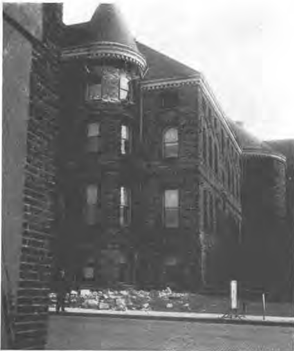
FIGS. 10 AND 11—Old State Building, Olympia. Heavy sandstone walls, weak mortar and lack of adequate anchorage contributed to this damage.
