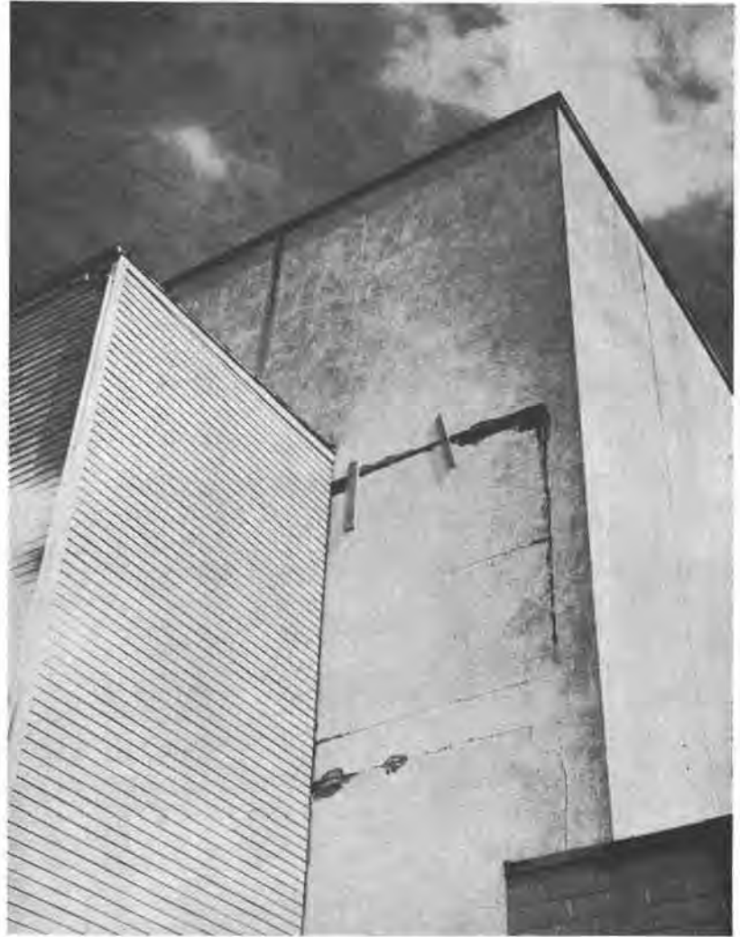
ON THIS SCHOOL building at Chehalis the action of the earthquake broke out the masonry filler walls in this concrete frame with complete separation from beams and column.
