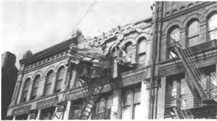
FIG. 4—Failure of parapet wall and collapse of fire escape. —Photo by U. S. C. & G. S.
