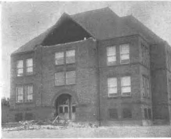
FIG. 4—Lafayette School in west Seattle. The gable fell because of lack of adequate anchorage and defective masonry. The masonry fell on the landing in front of the main entrance
