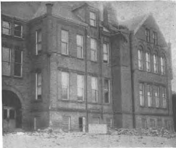
FIG. 5—Lafayette School, west Seattle. A large number of brick from the chimney fell in the school play-yard.
