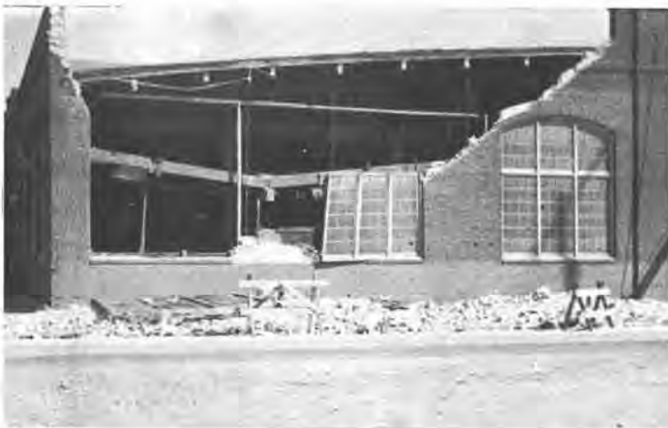
FIG. 5—Collapse of brick filler wall. This wall at the Crane Company, East Marginal Way and Hinds Street, Seattle, boiler and radiator shop, fell outward in the earthquake, saving workmen inside.—Seattle Times photo.
