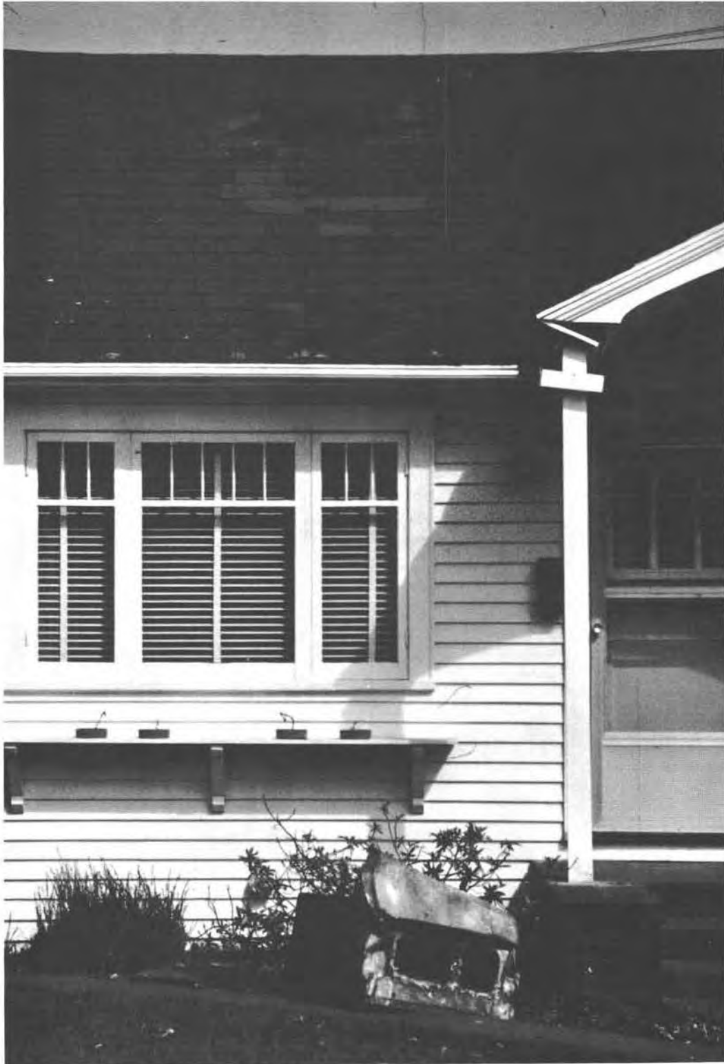
Figure 21.—Chimney damage in West Seattle. (Photo by Karl V. Steinbrugge.)
