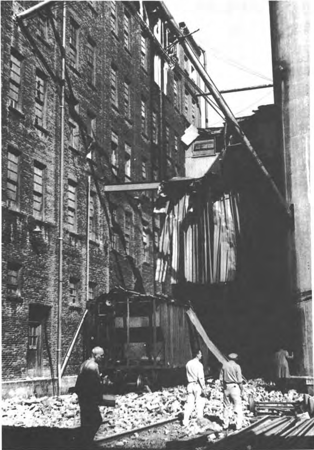
Figure 17.—Unreinforced brick fell from top story at Fisher Flouring Mills, Seattle. (Photo by John Vallentyne, Seattle Post-Intelligencer.)
