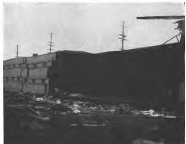
FIG. 3—This is a wood frame building resting on concrete piers. Apparently the foundation collapsed, allowing the floor to slope and catapult the contents of the building through the exterior wall.
