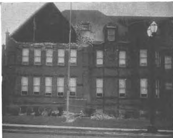
FIG. 6—Lafayette School, west Seattle. Gable and chimney fell due to weak masonry and inadequate anchorage.
