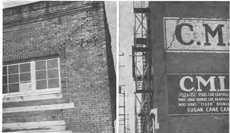
LEFT—Unsupported by any adjoining building, the corner of this structure moved out from under the roof the distance indicated by the crack.
