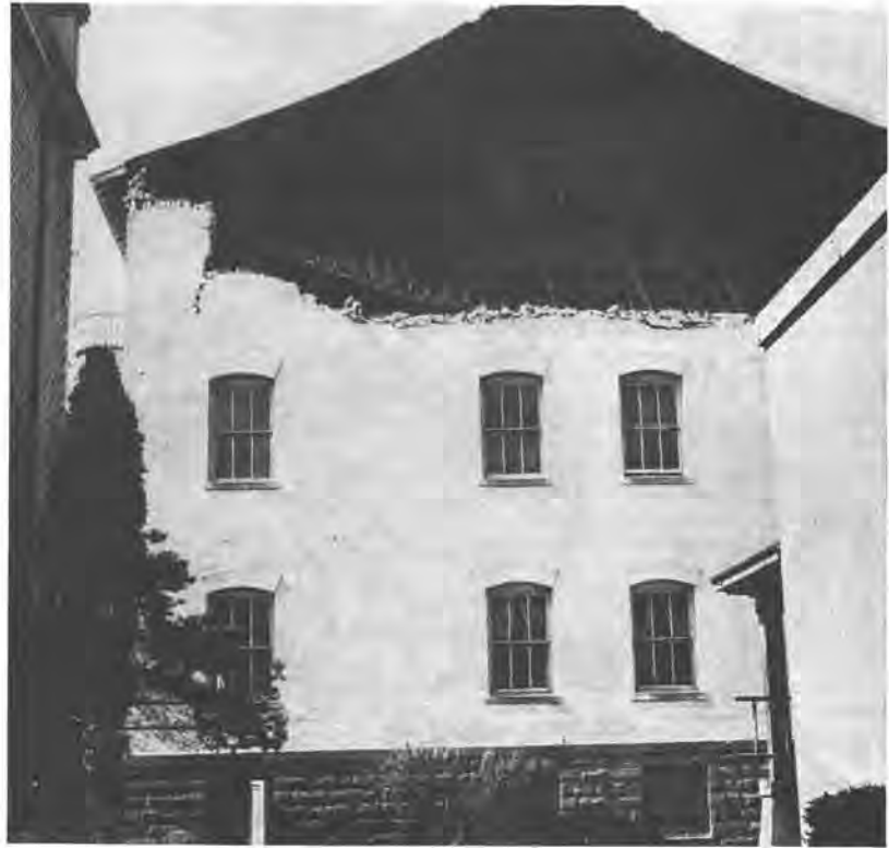
TYPICAL of pre-1900 buildings, this tall thin wall and unanchored gable were easily knocked out by flexing of wood structure. Crack to left shows side wall about to fail.
