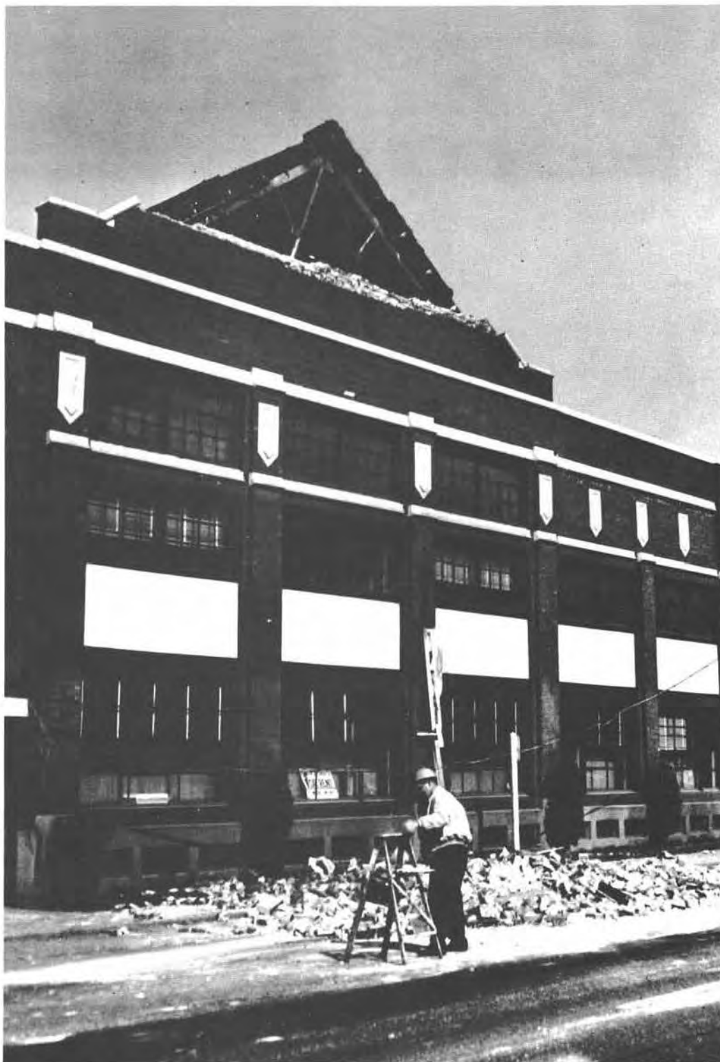
Figure 13.—Failure of an unreinforced brick gable in Seattle. The masonry fell on a parked car, injuring occupant (see Figure 14). (Photo by Seattle Fire Department.)
