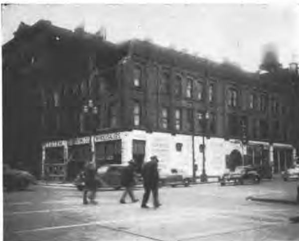
FIG. 2—This entire building is constructed with a very inferior grade of masonry, weak mortar and lack of joint filling. The parapet wall near the corner fell because of defective masonry and lack of anchorage.
