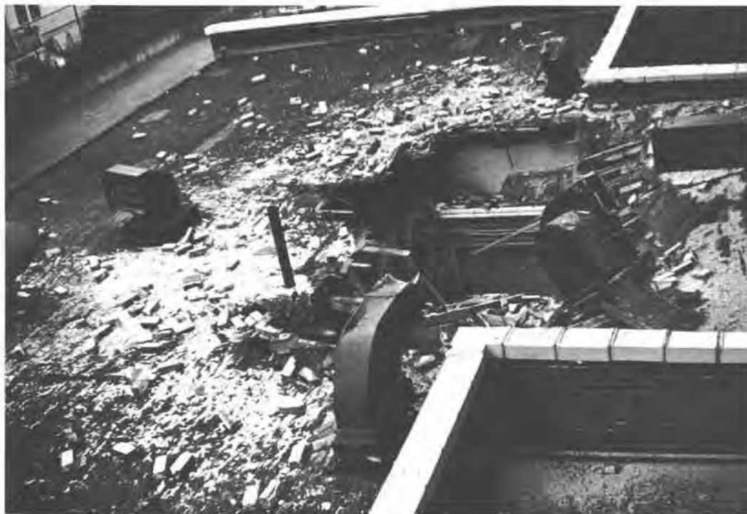
Figure 19.—Hole in the roof due to the collapse of the chimney shown in Figure 18. (Photo by Karl V. Steinbrugge.)
