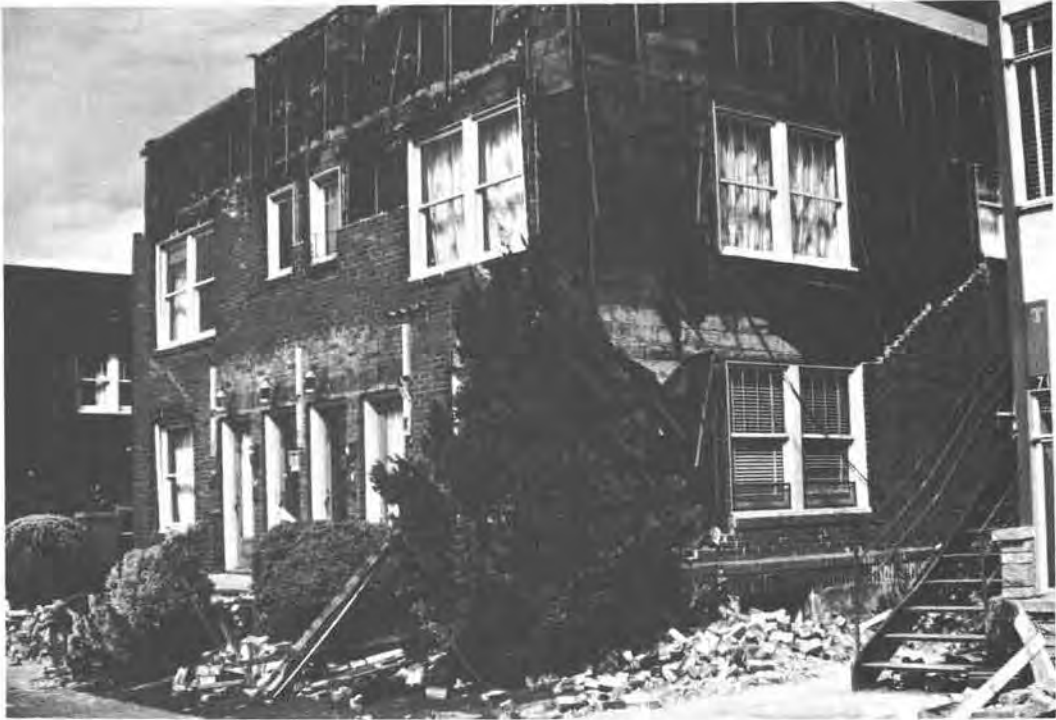
Figure 22.—Four-inch thick brick veneer peeled off of this wood frame structure in Seattle. The galvanized metal anchors were imbedded in a bed of low strength mortar. (Photo by Karl V. Steinbrugge.)
