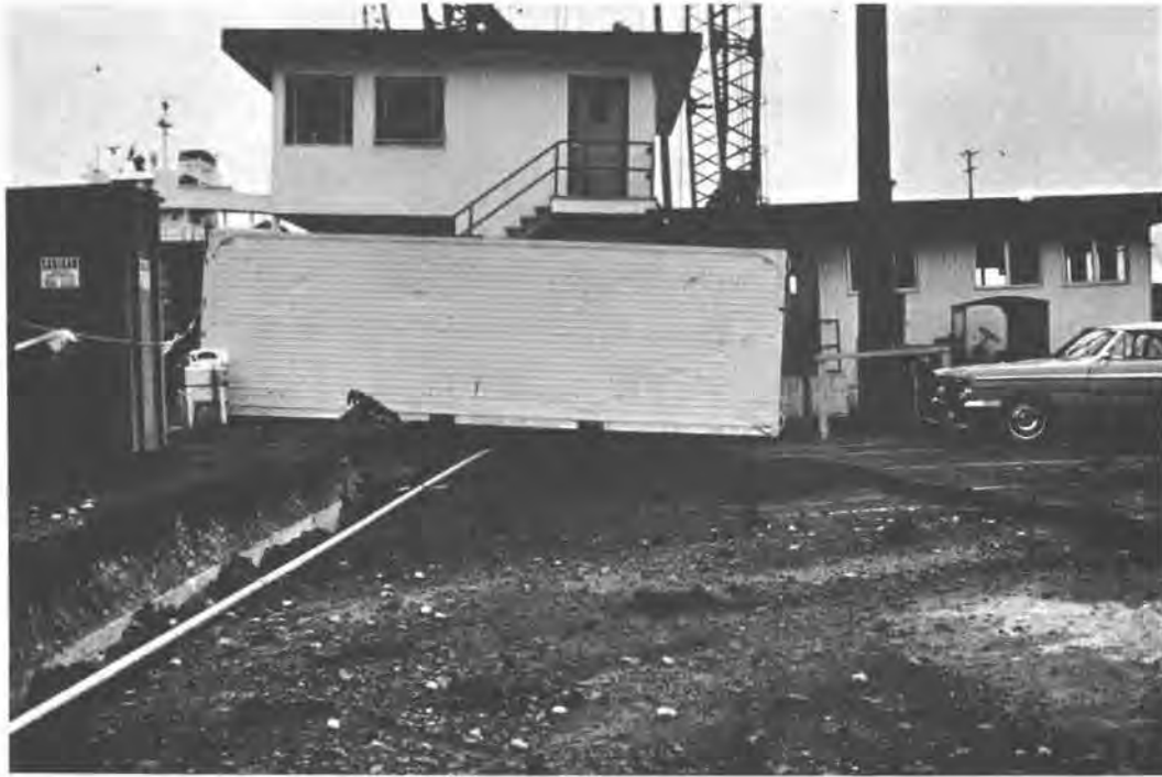
Figure 26.—Ground dropped due to the pier at the left shifting toward the water. Location is Harbor Island in Seattle. (Photo by Karl V. Steinbrugge.)
