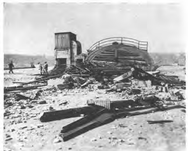
FIG. 6—Collapse of 54,000-gallon wooden tank on roof of six-story reinforced concrete cold storage plant at Seattle.—Photo by Harry Davis, Seattle.
