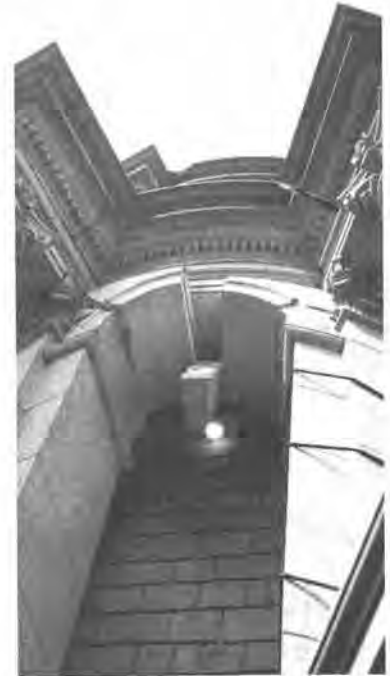
IN THE CAPITOL DOME at Olympia, erected in 1925, unanchored keystone dropped and column caps broke away. It takes strong mortar, steel and concrete, besides stone, to make such structures earthquake-resistant.
