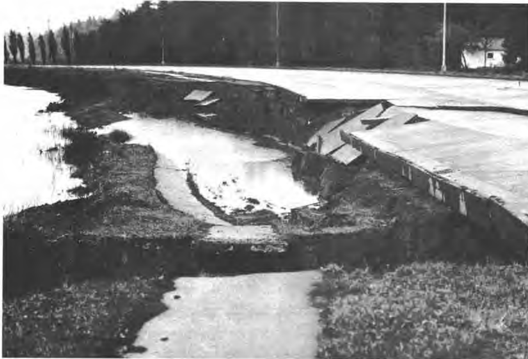
Figure 24.—Landslide damage to a roadbed in Olympia. (Photo by Karl V. Steinbrugge.)
