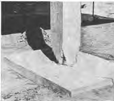
CONNECTIONS between structures must be rigid enough that both structures move as a unit or be separated so they move independently. Above, damaged base of an unbraced column.
