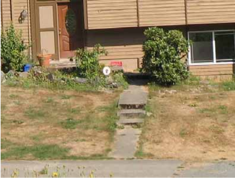
Figures 5-11: Unscreened, raised wooden porches and decks can accumulate flammable material underneath.
