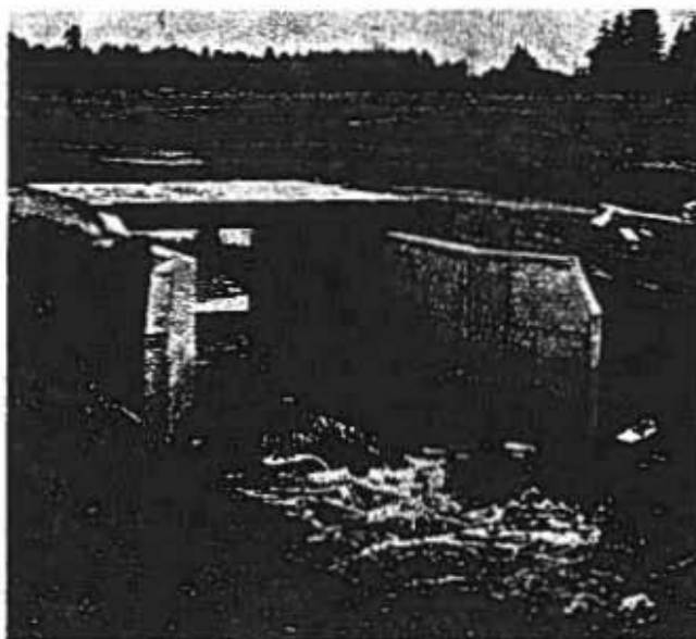
PHOTO 22-21. Fishway on Blooms Ditch diversion dam.
