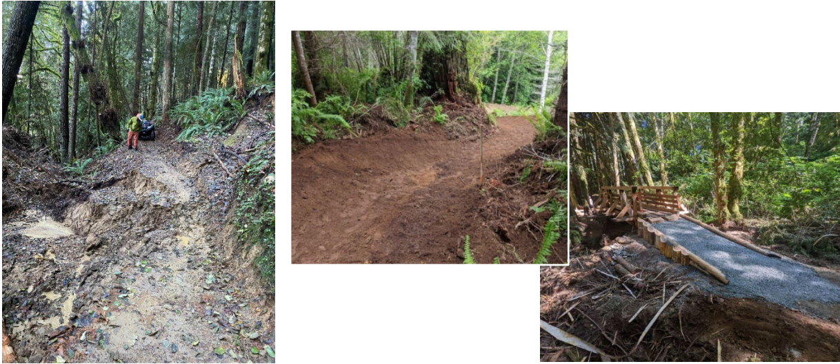
Sadie Creek Lyre River section slide (left), Sadie Creek Highpoint Trail (middle), Sadie Creek Highpoint Trail Bridge (right).
