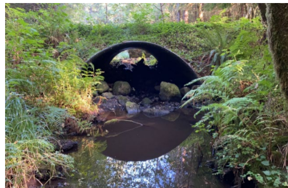
Typical fish passable culvert. Photo: Alex Nagygyor
