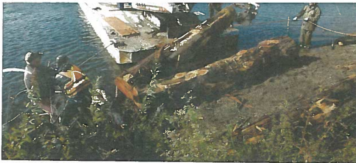
Journal photo by Gordon Weeks Volunteers and Taylor Shellfish employees last Friday unload huge cedar logs onto the island in the middle of Island Lake. The logs, gravel and 900 new plants and trees will restore the shrinking island.
