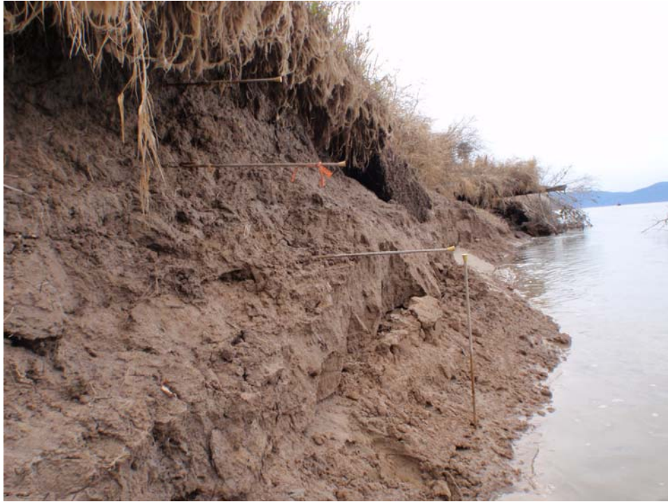
Figure 20. Bank Erosion in the Clark Fork River Delta. Photo taken on November 16, 2009. Bank pins were put in on April 8, 2008. 2.6 feet now exposed. Photo Courtesy of Kathy Cousins (Idaho Department of Fish and Game)
