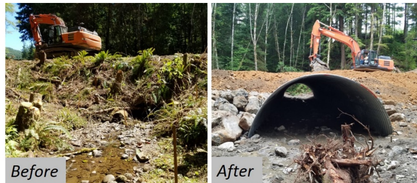
Figure 6-1: Fish-Barrier Removal on an Unnamed Tributary to Kalaloch Creek. This project replaced a 60-inch corrugated metal pipe (left) with a 16-foot-diameter multi-plate culvert (right). A total of 0.7 miles of salmon and trout habitat were opened up as a result of this project. Photos courtesy of Jeremy Tryall.
