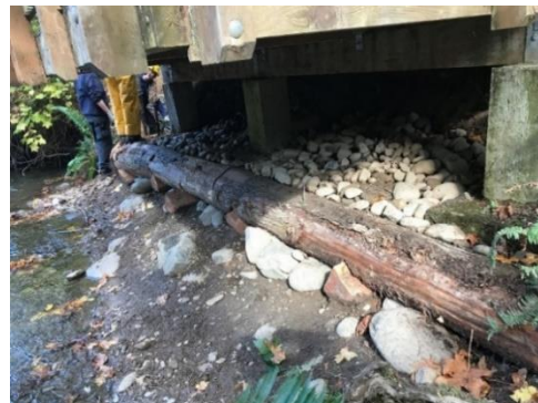
Figure 21: A Cedar Crib Log Was Used to Stabilize a Fishing Platform at the Lyre River Campground. Photo courtesy of Justin Zarzeczny.
