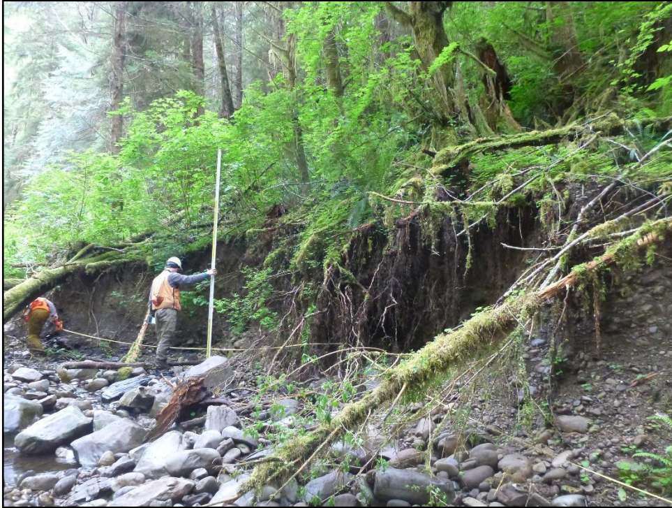
Figure 2-8. Field crew measuring active erosion height and length.
