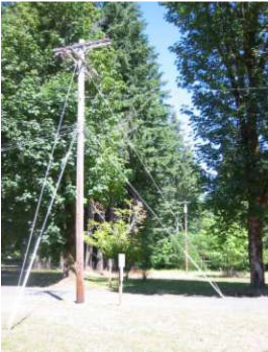
Figure 5. Power lines broken by a tree caused the 2003 Herman Creek Fire (Image: S. Zielin, Skamania County).
