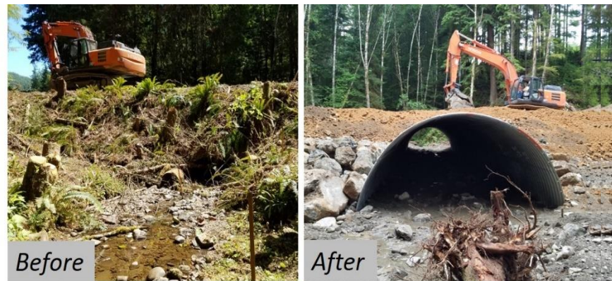
Figure 6-1: Fish-barrier removal on an unnamed tributary to Kalaloch Creek. This project replaced a 60-inch corrugated metal pipe (left) with a 16-foot-diameter multi-plate culvert (right). This project opened up a total of 0.7 miles of salmon and trout habitat. Photos courtesy of Jeremy Tryall.
