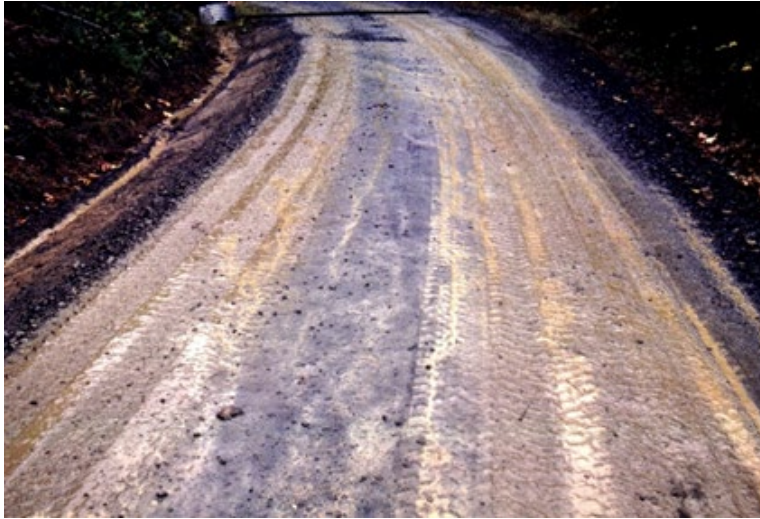
Figure 8. An example of a wet forest road surface after trucks have passed. The sediment in the upraised patterns are fine sediments that were pressed into tire sipes and would be easily transported if it were raining.
