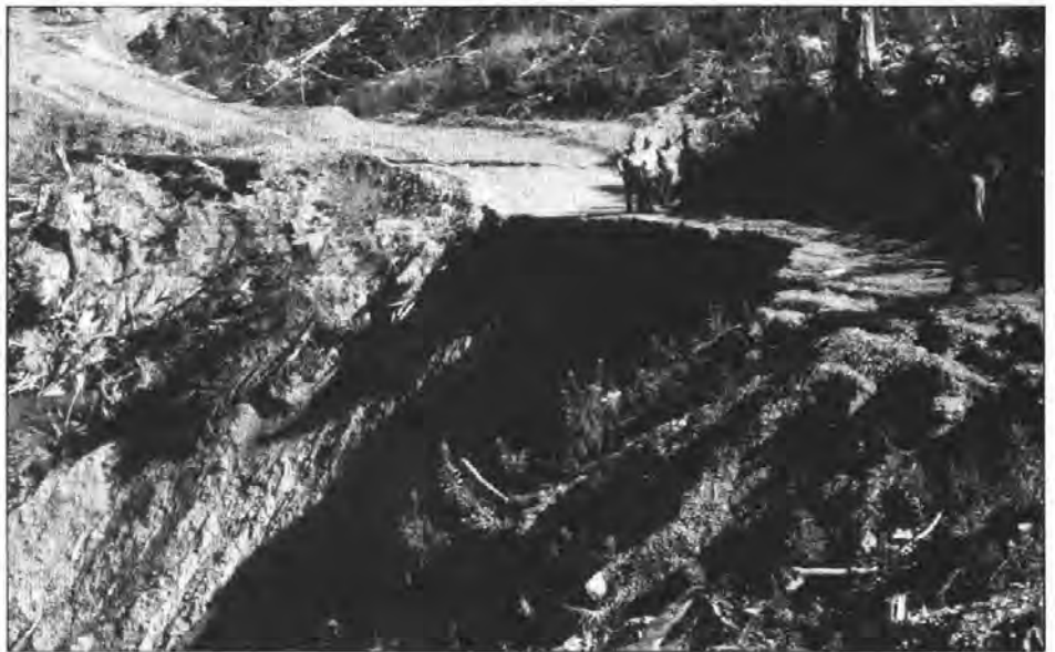
Figure 4. Road damage like this is typical of the aftermath of an earthquake. Four-wheel drive is seldom of benefit in such a setting. Travel at night in these situations can be especially hazardous.
