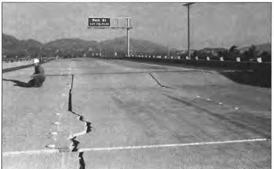
Figure 5. Bridge-approach fills commonly compact and settle during an earthquake, even though the bridge itself may be undamaged. Here, settlement has created a 'launching ramp' for cars. Elsewhere, settlement can create vertical concrete walls. This example is from the 1971 San Fernando, California, earthquake.
