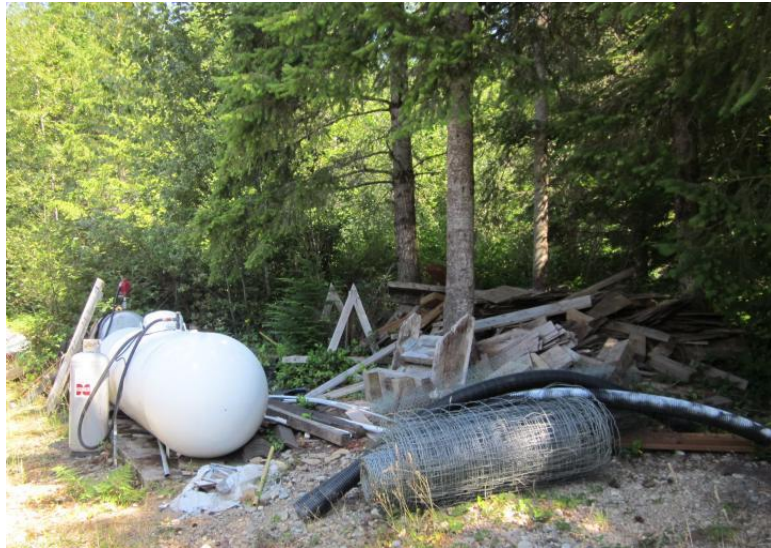
Figure 5-12: Above ground propane tank with nearby flammable materials.
