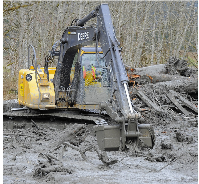
An Excavator Working in the Debris Field near Oso. Photo courtesy of WSP. Flickr/Snohomish County - CC: BY-NC-ND 2.0
