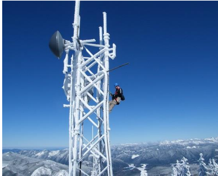
A Technician Repairs Microwave Dishes on a Communication Tower Located on State Trust Lands (Grass Mountain, South Puget HCP Planning Unit). Photo: Steve Diamond, NorthWest Tower Engineering, Inc.
