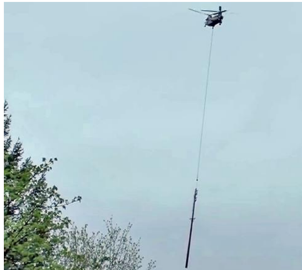
Chinook Helicopter Transports a Replacement Structure to a Remote Portion of a Transmission Line Photo: Bonneville Power Administration
