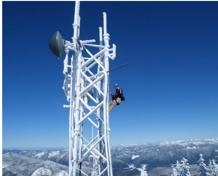
A technician repairs microwave dishes on a communication tower located on state trust lands (Grass Mountain, South Puget planning unit). Photo: Steve Diamond/NorthWest Tower Engineering, Inc.
