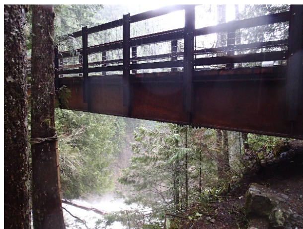
Figure 21: Non-Motorized Trail Bridge over the Wallace River in Reiter Foothills Forest. Photo courtesy of Jim Patton.
