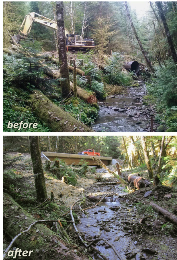
Figure 17: Tributary to Christmas Creek in the OESF. This project replaced an existing 72" corrugated metal culvert with a 60' bridge, opening approximately 1.5 miles of previously obstructed Coho, steelhead, and cutthroat habitat. Photos courtesy of Candace Montoya.
