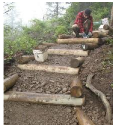
These box steps were built as part of a trail restoration project and will help minimize erosion by providing a stable and water-permeable hiking surface.
