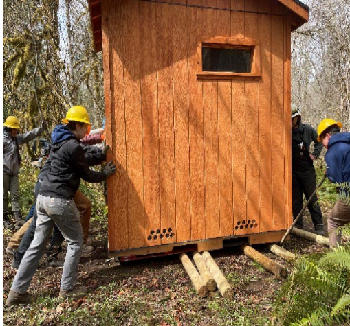
WCC and PC Recreation Staff install new outhouses at Winston Creek. Photo: Sharon Steriti
