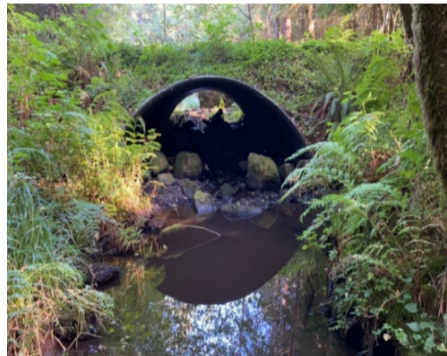
A fish passable culvert which does not require correction. Photo: Alex Nagygyor
