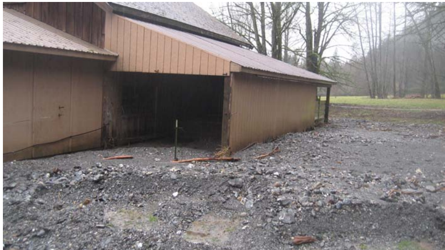
Figure 13 Debris against barn walls, Stavik property. View looking northwest. (Hooks, 2009)
