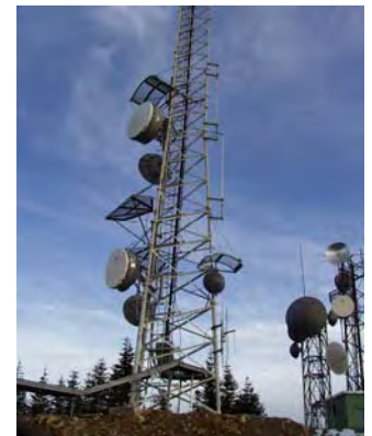
A communications tower on DNR-managed land.
