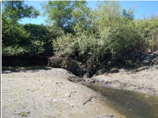
Debris over Culvert Outlet
