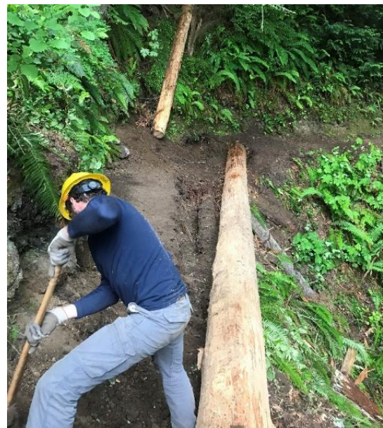
Figure 24: Repair Work on the Striped Peak Trail. Photo courtesy of Justin Zarzeczny.
