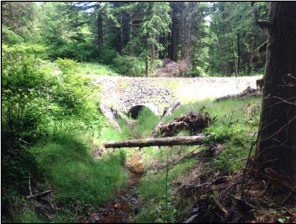
Figure 1. A reconstruction project on a Type 3 stream with placed wood downstream of the crossing. This crossing has a log spanning the stream as well as logs and detached root wads placed adjacent to the stream within the inner zone.
