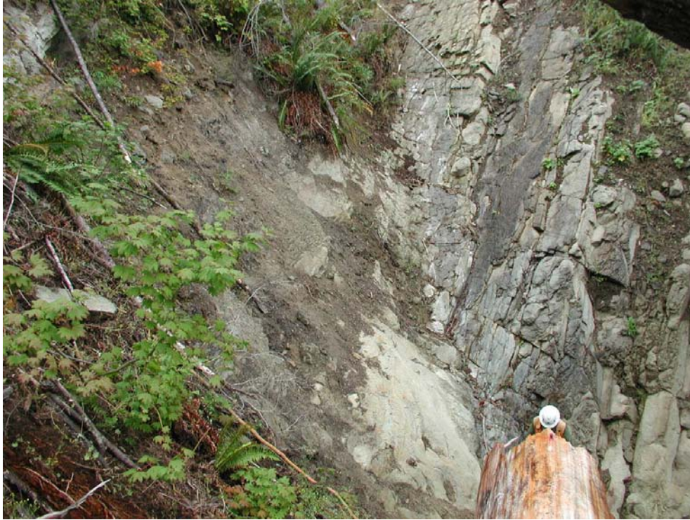
Figure 4 Main Bittner Creek PI. Soil layer and organic debris slid off of bedrock surfaces on both sides of channel. View looking east. (Coyle, 2009)
