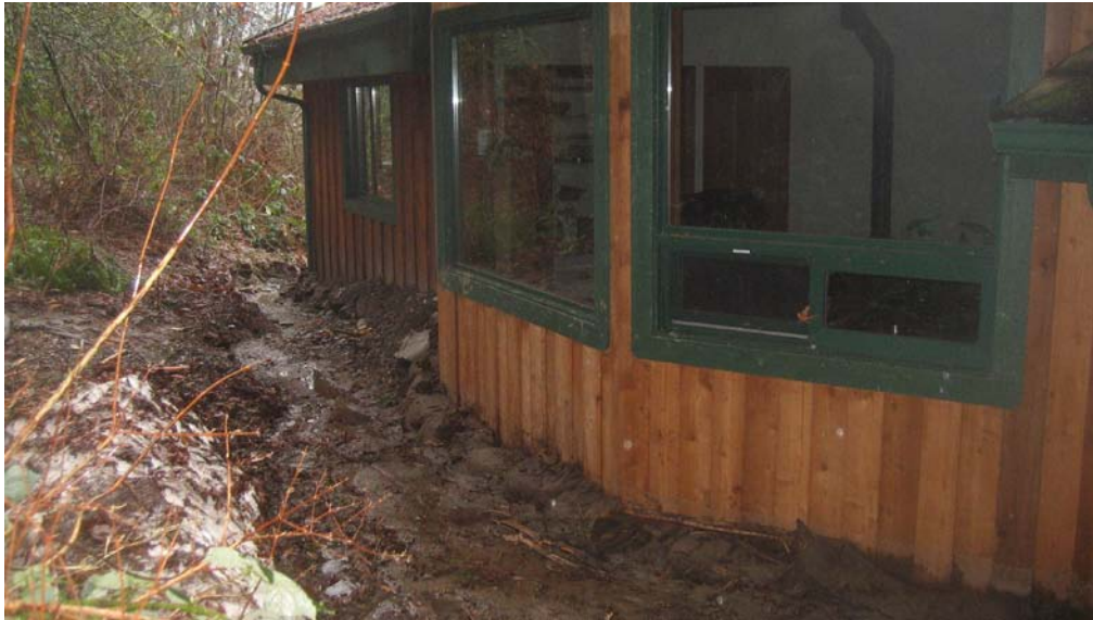
Figure 8 Debris flood deposition along the east side of the residence at 3334 Clipper Road. View looking south. (Hooks, 2009)
