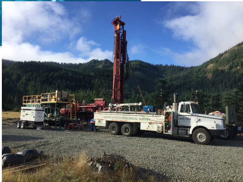
Figure 11. Geothermal drilling near Mount St. Helens. Lidar was an input for the original modeling work, and was also used for drill site planning.
