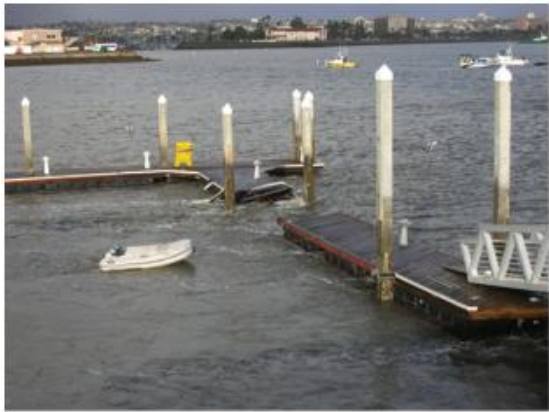
Figure 9. Docks were destroyed and boats pulled from moorings at Shelter Island in San Diego Bay during the February 2010 Chilean tsunami. ♦
