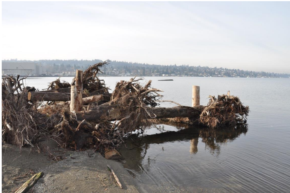
FIGURE 3.— Photo of a newly constructed engineered logjam (ELJ-A, January 15, 2015). From January to June, the lake level rises approximately 0.6 m to inundate much of the logjam shown.
