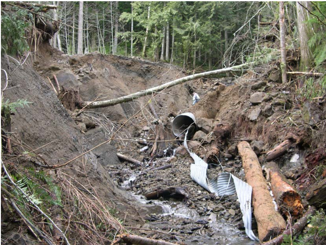
Figure 5. Photograph of Washed Out D-6200 Road. Photograph taken facing north.
