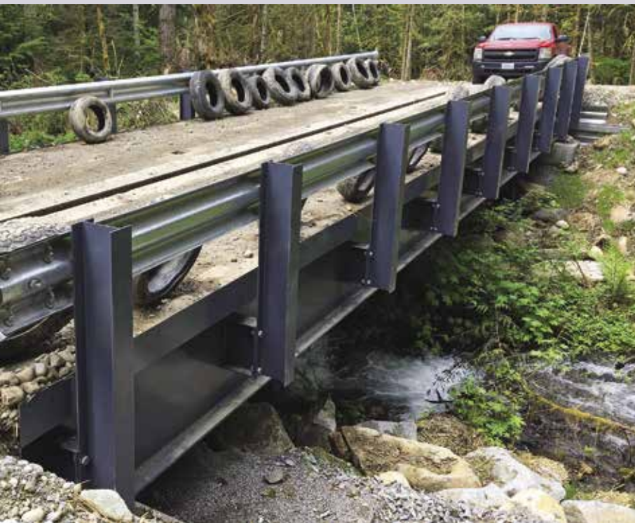
A bridge wide enough to support fish passage was installed as part of the Turning Wheel Timber Sale process.
