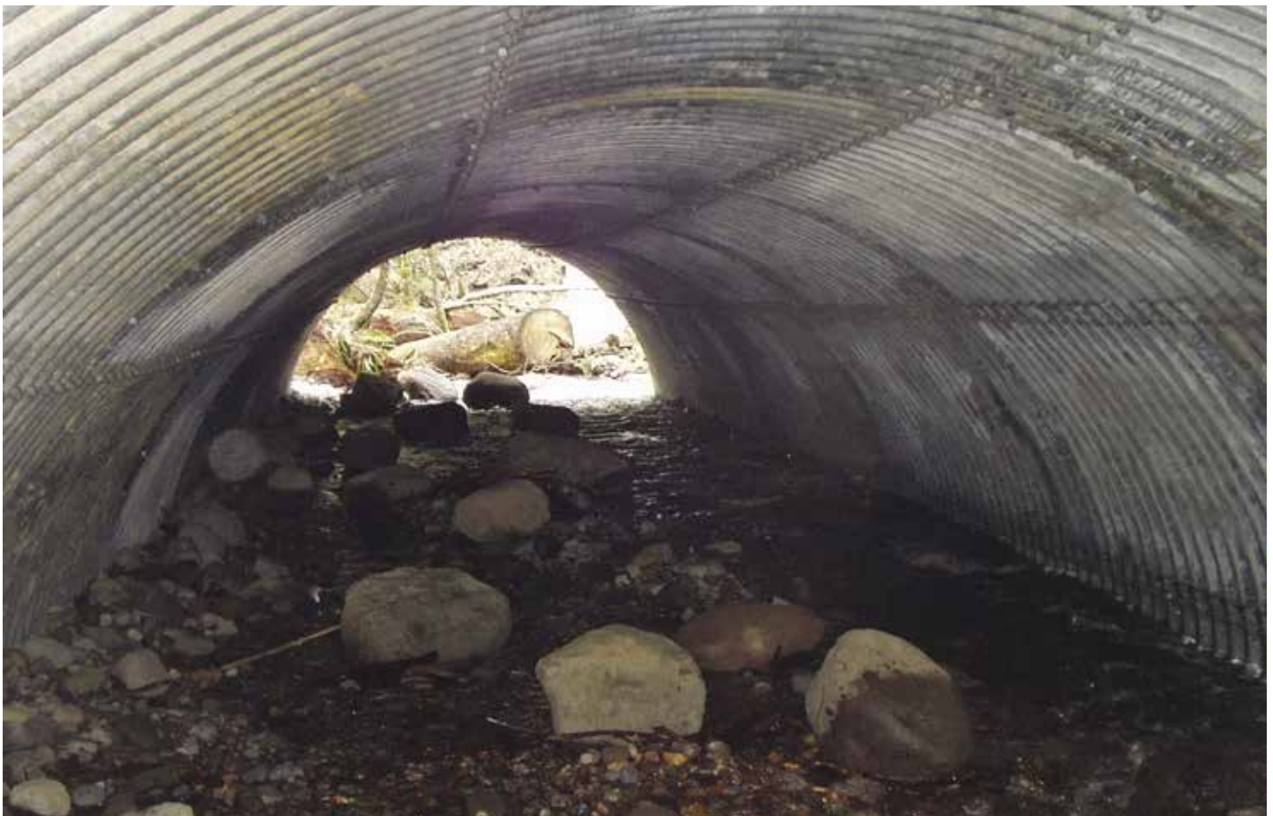
Stream simulation culverts support fish passage.
