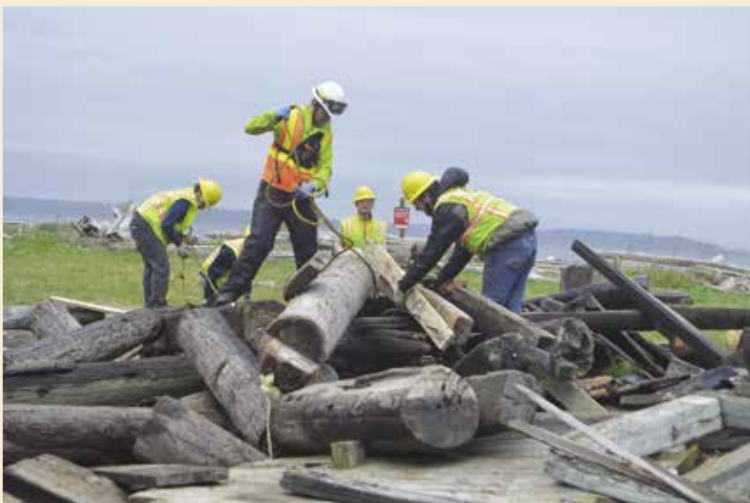
Workers construct an engineered log jam as part of a beach restoration project.
