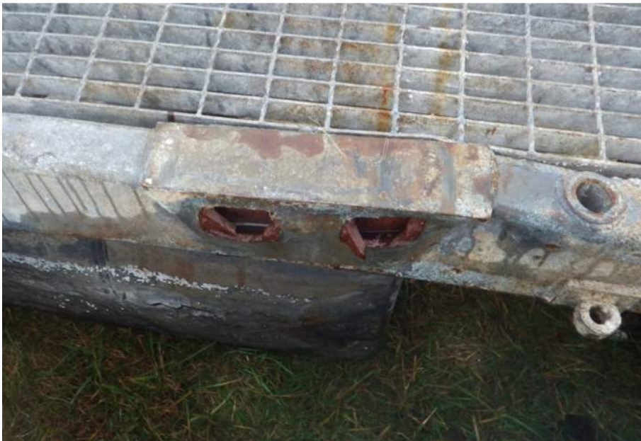
Figure 7.12 – Broken Hinge Connection on Catamaran Float at location of Main Bridge Float (Source: Mott MacDonald)
