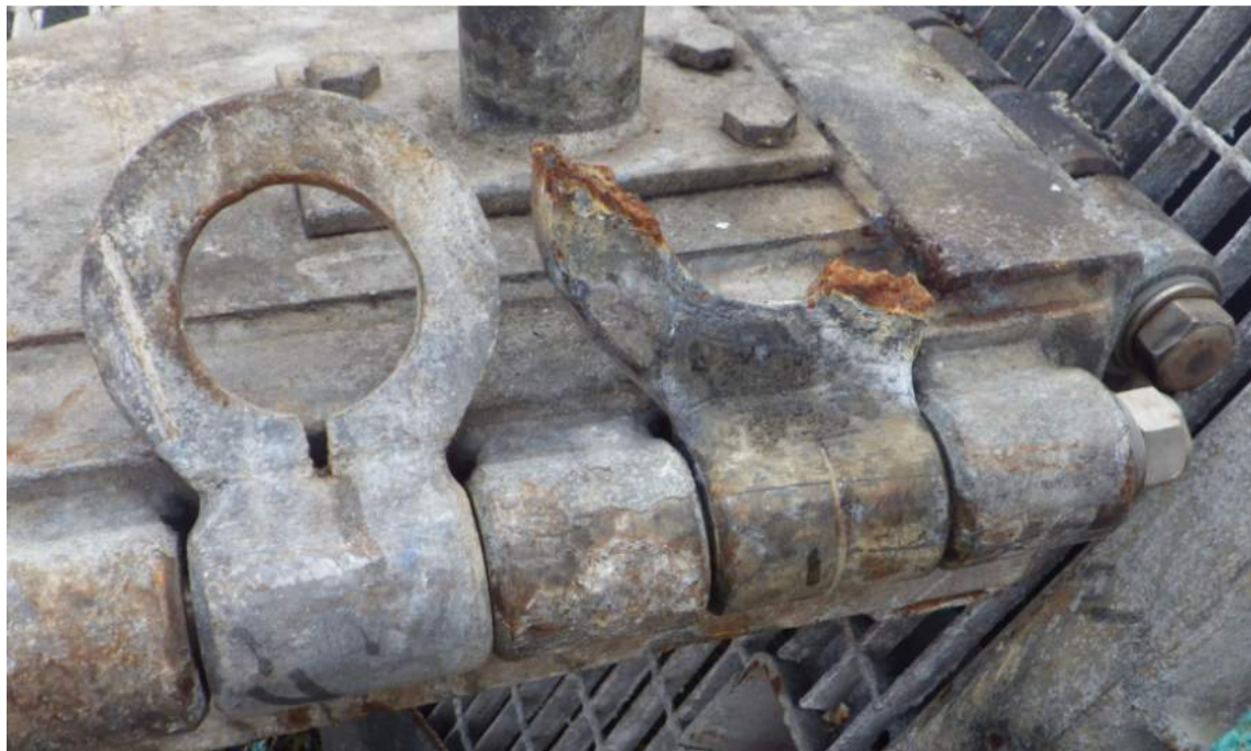
Figure 7.9 – Failed Pad Eye (Source: Mott MacDonald)
