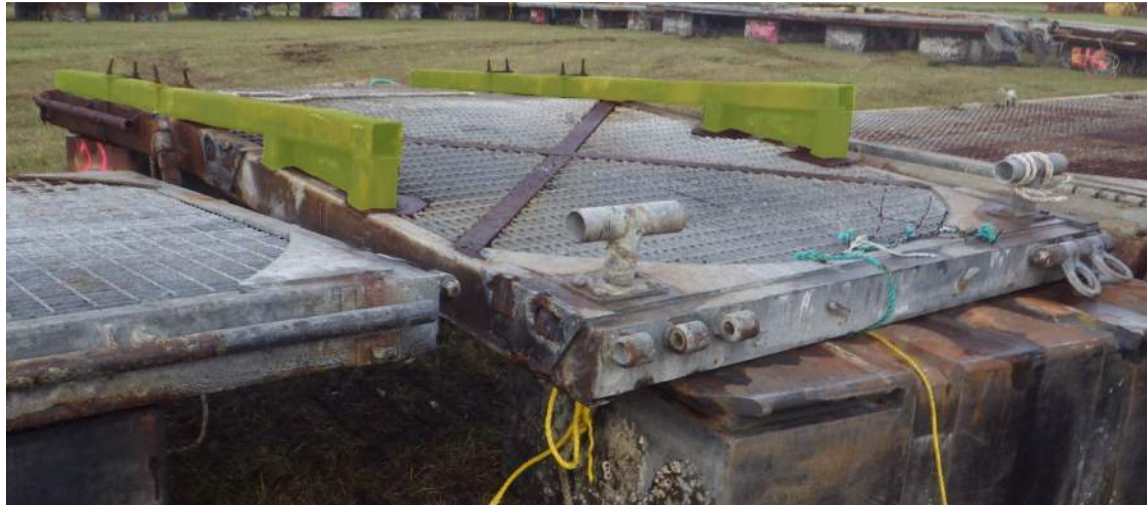
Figure 7.10 – Repairs to floats following July 2017 incident (shown in yellow) Cross-bracing on the surface of the floats was installed earlier in the life of the net pen structure. (Source: Mott MacDonald)
