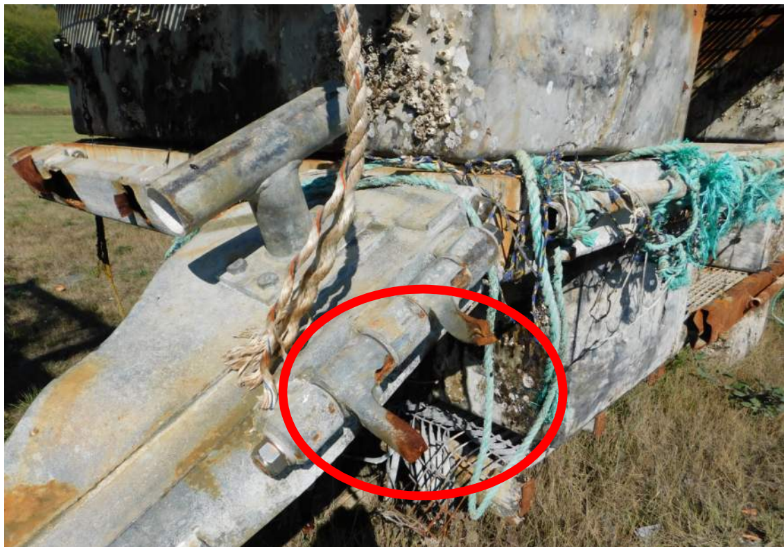
Figure 7.5 – Broken pad eyes on an Outrigger Float (Source: Mott MacDonald)
