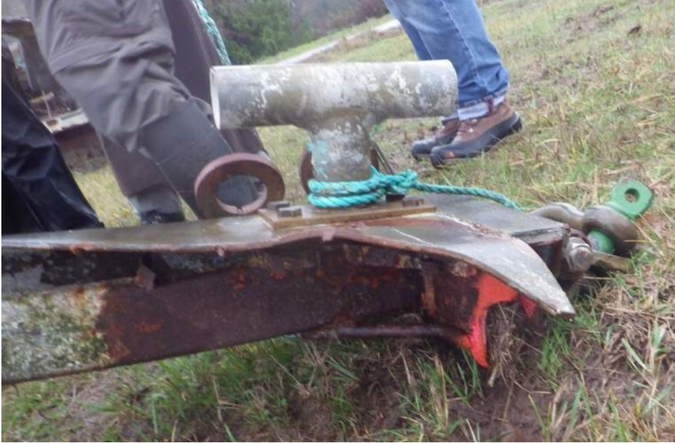
Figure 7.14 – Broken Structural Framing Member at Corner of Outrigger Float – Northeast Corner of pen 225 (Source: Mott MacDonald)
