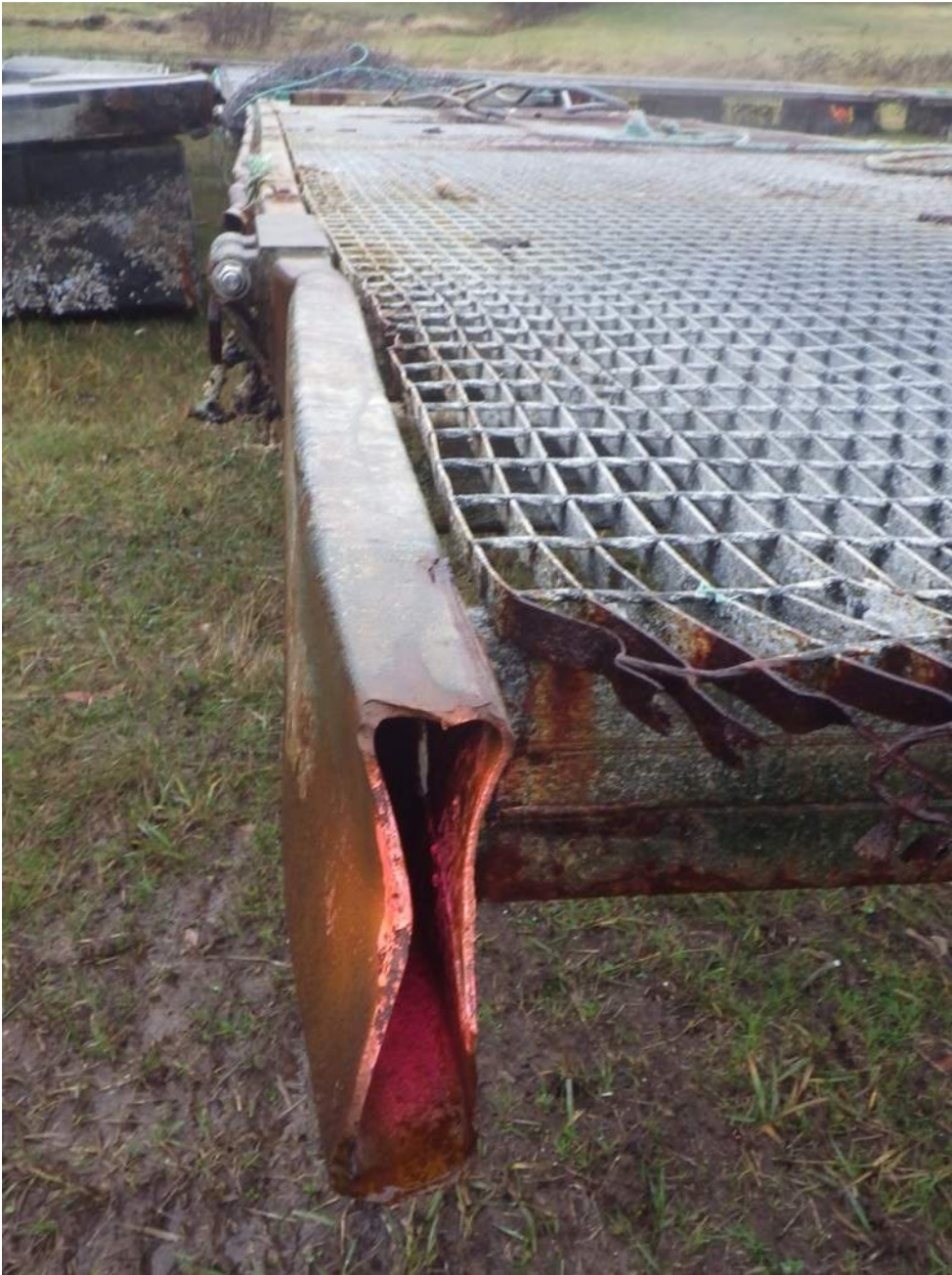
Figure 7.13 – Broken Structural Framing Member on Outrigger Float (Source: Mott MacDonald)
