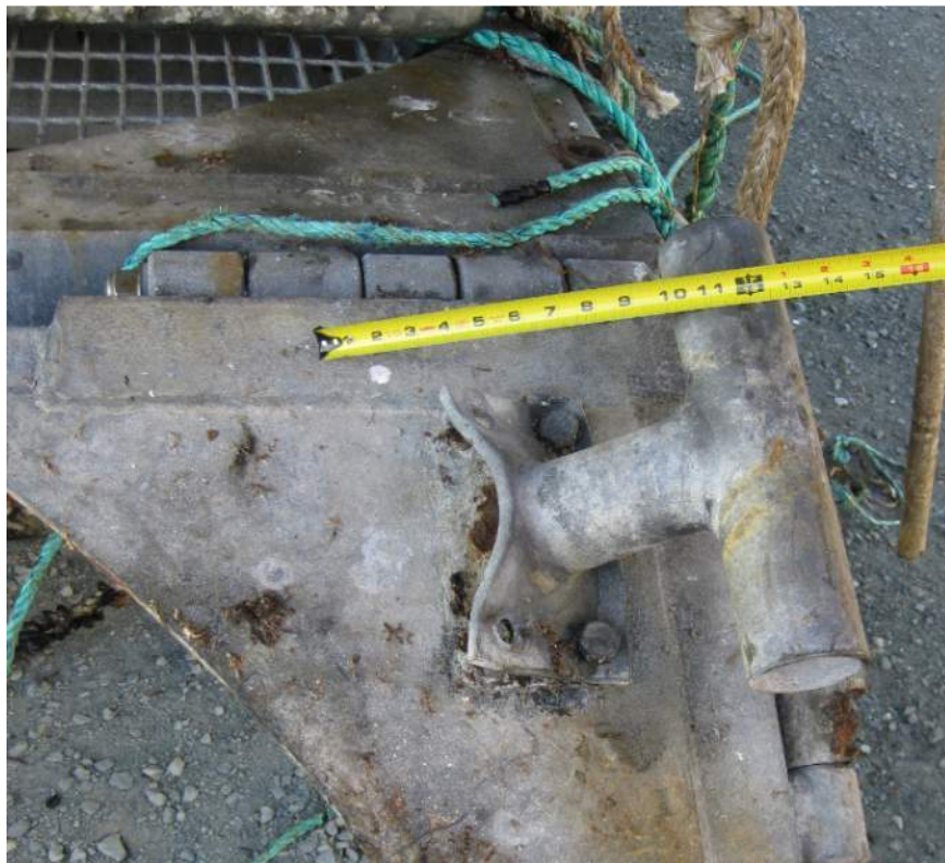
Figure 7.4 – Bent mooring cleat on an Outrigger Float (Source: Mott MacDonald)
