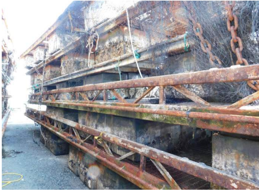
Figure 7.3 – Floats showing corroded framing (Source: Mott MacDonald)
