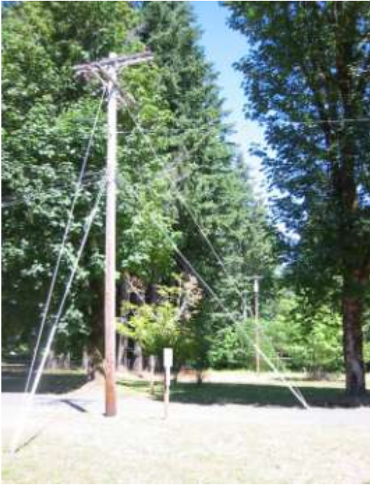
Figure 6. Power lines broken by a tree caused the 2003 Herman Creek Fire (Image: S. Zielin, Skamania County).
