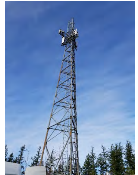
IMAGE SHOWS A COMMUNICATION TOWER LOCATED AT THE SUMMIT LAKE COMMUNICATION SITE ON STATE TRUST LANDS. SOURCE: WA STATE DNR
