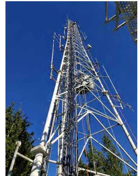
IMAGE SHOWS A COMMUNICATION TOWER LOCATED AT THE GOLD MOUNTAIN COMMUNICATION SITE ON STATE TRUST LANDS. SOURCE: WA STATE DNR
