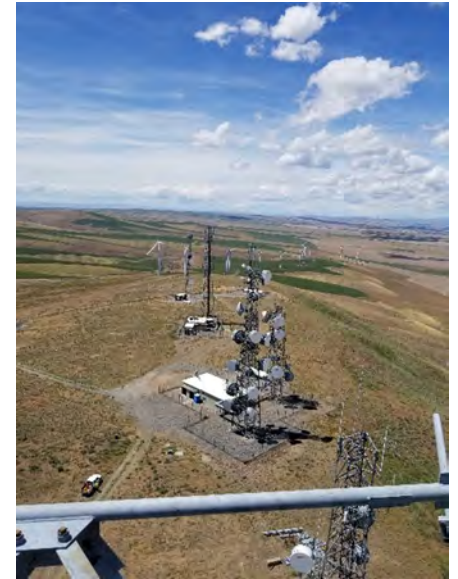
IMAGE SHOWS THE JUMP OFF JOE COMMUNICATION SITE LOCATED ON STATE TRUST LANDS. SOURCE: WA STATE DNR
