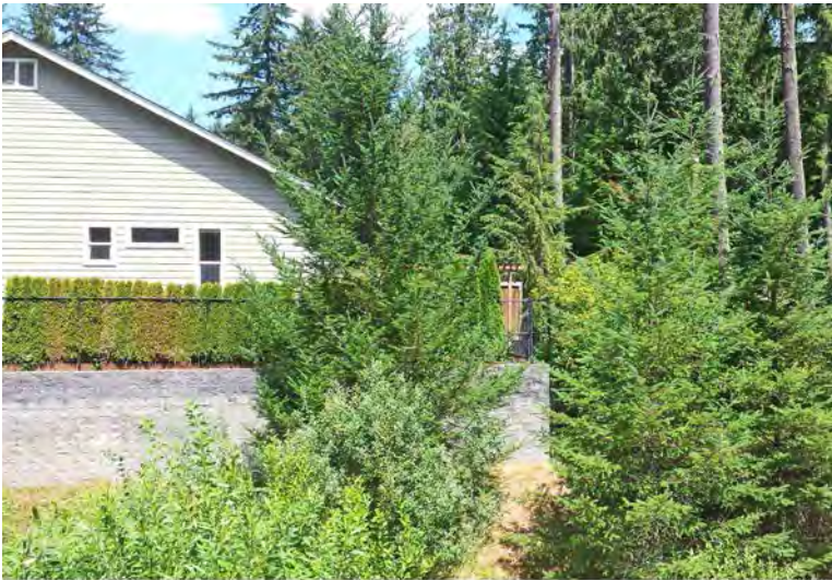
Figure 5-14: Even when located away from a residence, resinous plants can quickly spread flames between plantings, catching other fuels on fire. Note dead plants in the privacy hedge near the house.
