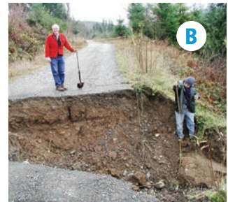
A Trees with pistol-butts (curved) can indicate the soil may be unstable and therefore unsuitable for road building.
